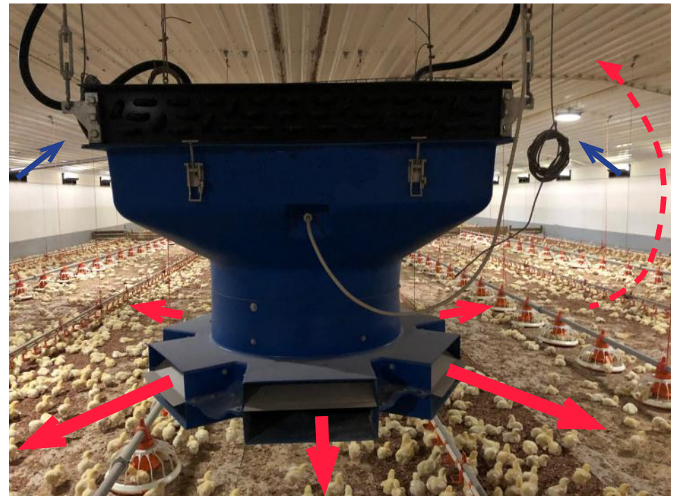
An illustration of a vertical circulation fan system. The thick red arrows show high velocity distribution and a thinner dashed red line shows the return air going back to the ceiling. The thick blue arrows indicate the cold air coming in through the perimeter inlets.
