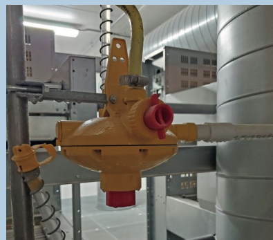
Flushing system (water regulator)
