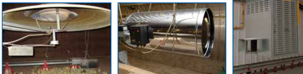
Figure 98: Examples of different house heating systems (from left to right, canopy brooder, whole-house heating, and space heater).
