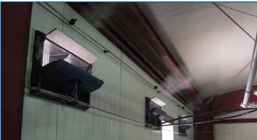
Figure 118: Example fogging system for a cross-ventilated house.
