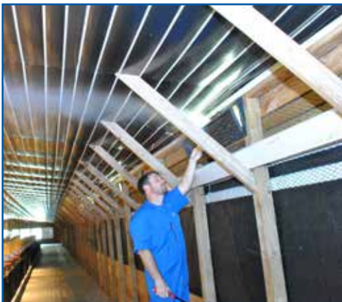
Figure 106: Using a smoke test to determine if air flow and operating pressure is correct.
