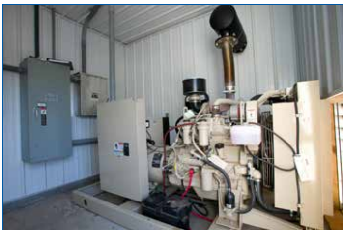
Figure 97: Example of a back-up generator.
