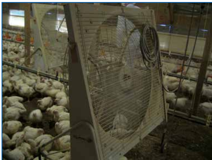
Figure 100: Circulation fans in a naturally ventilated house.
